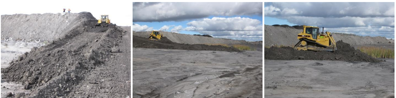
Figure 29: Start of pushing by D6 Swamp Dozer initial 1m thick capping layer of coarse reject over upper tailings beach
